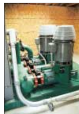
This set of variable frequency drive pumps allows maximum flexibility in irrigating the entire course in the shortest period of time, improving efficiency and reducing energy cost.
