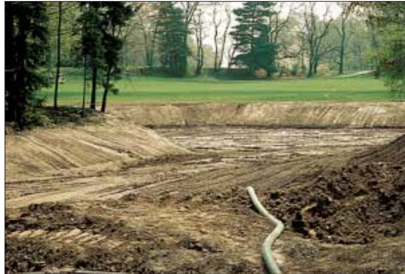
A 12 million gallon retention pond is being built on this golf course to collect surface runoff and subsurface drainage water for supplemental irrigation..
